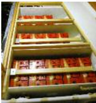
144 v battery bank
